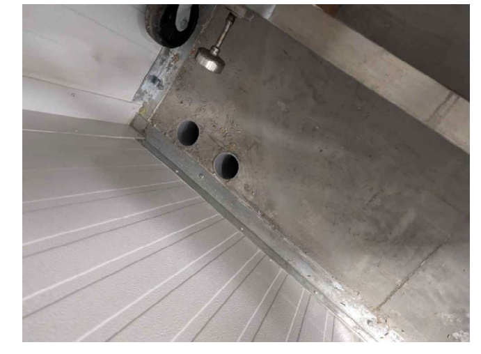
EXISTING 3.0" PARALLEL SERVICE FEEDER CONDUITS LOCATED IN PHASE 1 BREWING TENANT COOLER FLOOR AS SHOWN. CONDUIT HAVE BEEN CUT FLUSH TO FLOOR SLAB (SEE IMAGE ABOVE FOR EXISTING CONDITIONS). SLAB WILL NEED TO BE CHIPPED AWAY TO ALLOW CONDUITS TO BE EXTENDED INTO A JUNCTION BOX AND THRU WALL TO FEED PROPOSED PANEL MDP LOCATED IN PHASE 2. CONTRACTOR MUST COORDINATE PENETRATION LOCATION THRU EXISTING CONCRETE WALL PANEL WITH CONCRETE WALL PANEL MANUFACTURER.
